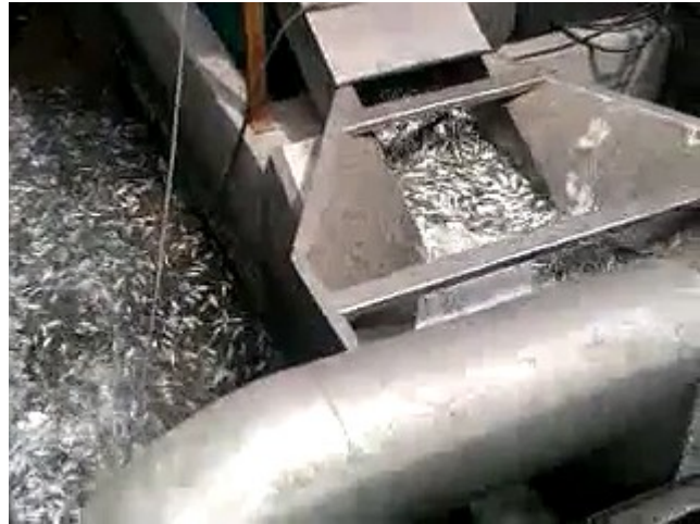
Fish entering the cooling system of the ZETES plant. (Image: Bartin Platformu)
