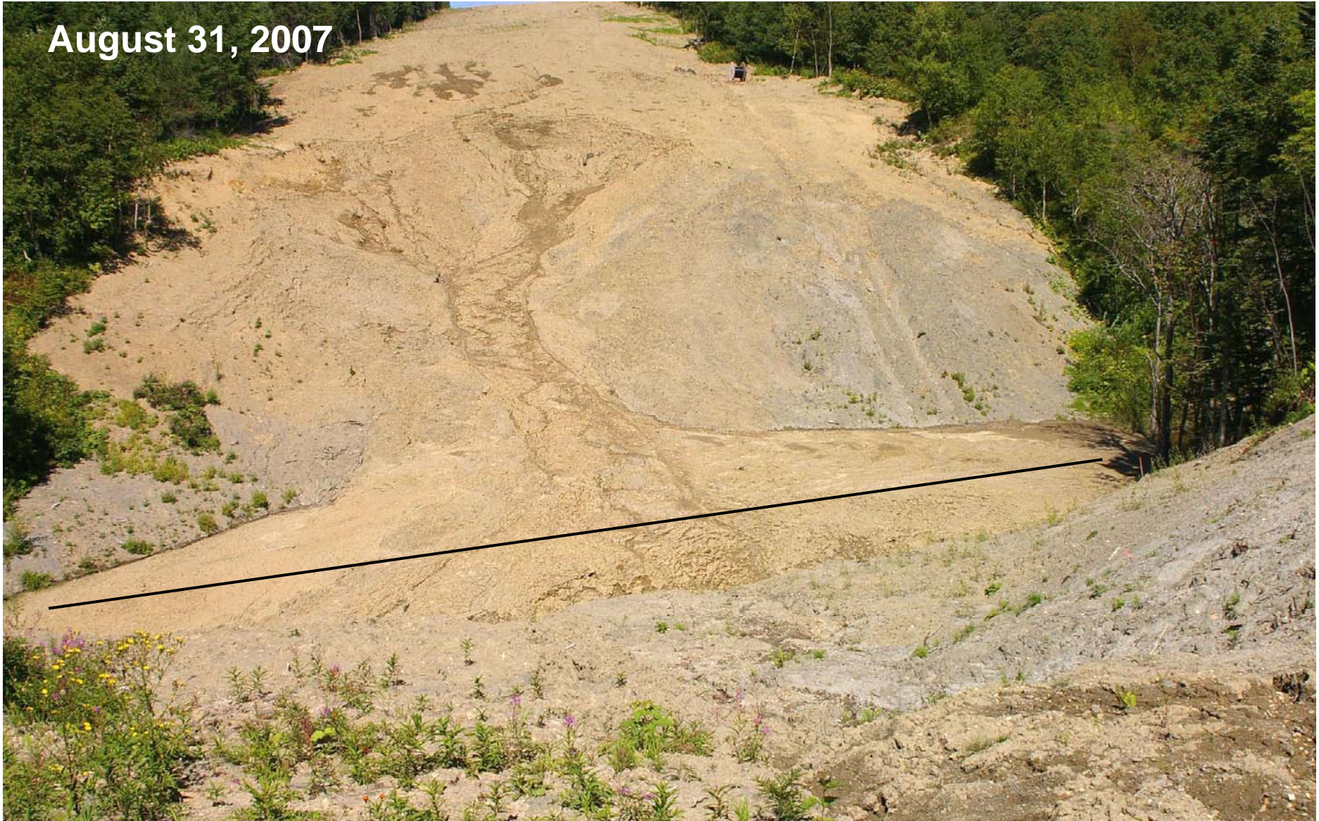
KP 462,6. The landslide on the right bank of the left tributary of the Baklanovka River, Dolinsk District.
