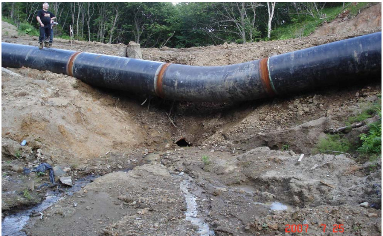
Un-numbered stream, tributary of Krinka River of the 2 nd order. KP 350.0. The culvert does not correspond to design requirements and matching conditions. The hydrological process of the water flow has been disrupted. Waste construction soil is entering the streambed and contaminating the water.
