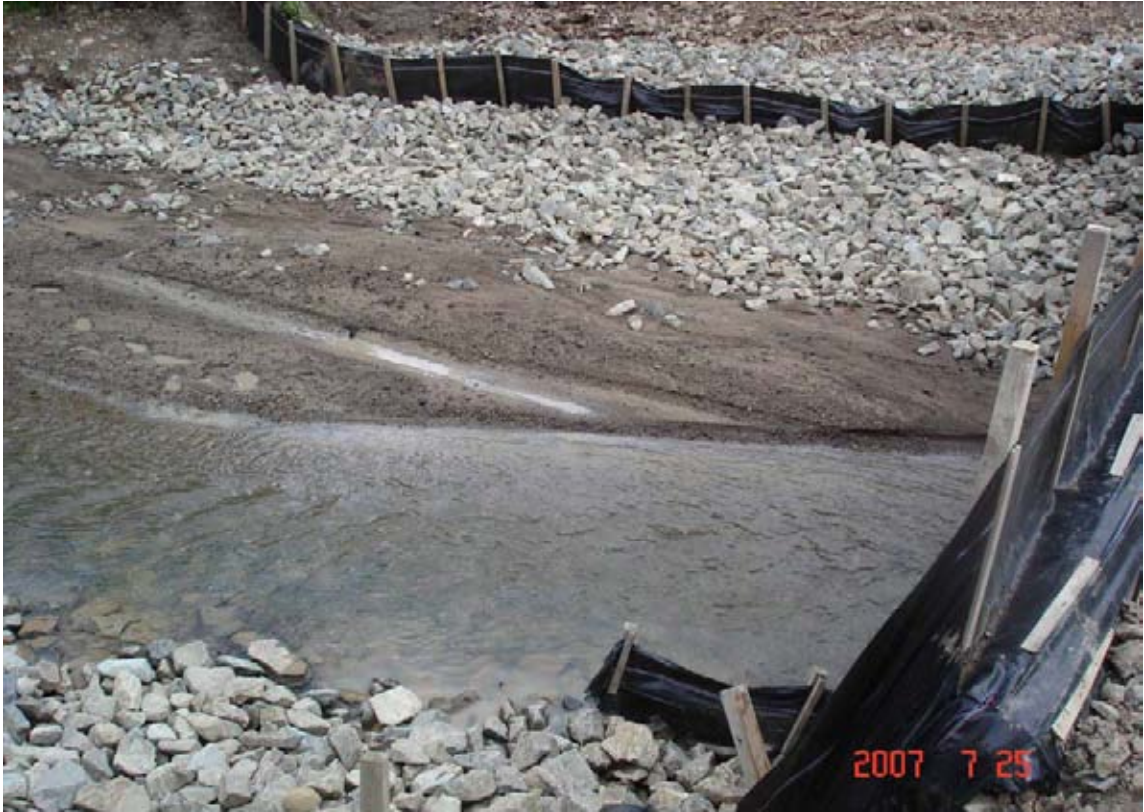
Krinka riverbed in the range of the gas pipeline crossing. July 25, 2007. In violation of the requirements of the project and responsibility of the company "Sakhalin Energy," the riverbed, where spawning grounds used to be located, the backfill consists of crushed stone instead of pebbles or gravel. In the center of the photograph sludge sediments are already visible above the crushed stone backfill. The presumed source of the sediments is the access road and the waste construction soil from the upstream pipeline route.
