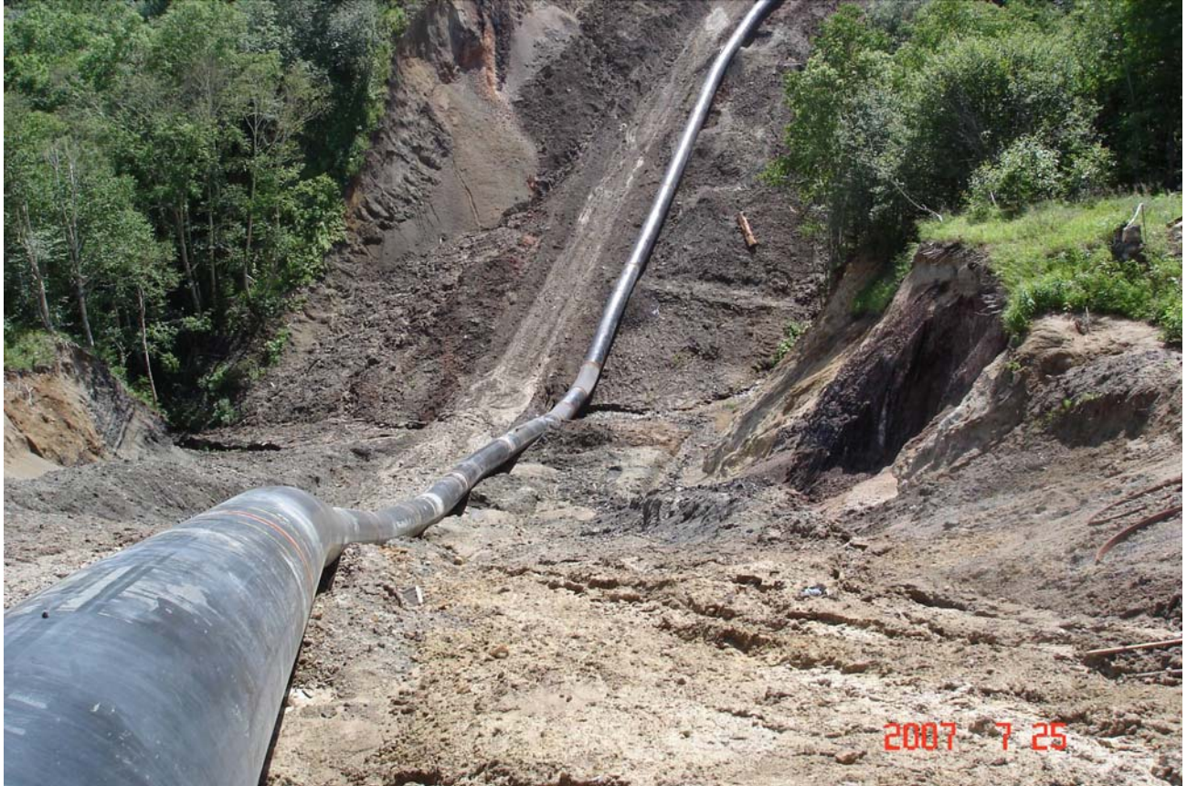
Petrovskii Stream, KP 351.1. A general view of the pipeline route stream-crossing. Anti-sludge screens and bank-stabilizers are absent. Erosion wash-outs are visible in the foreground.
