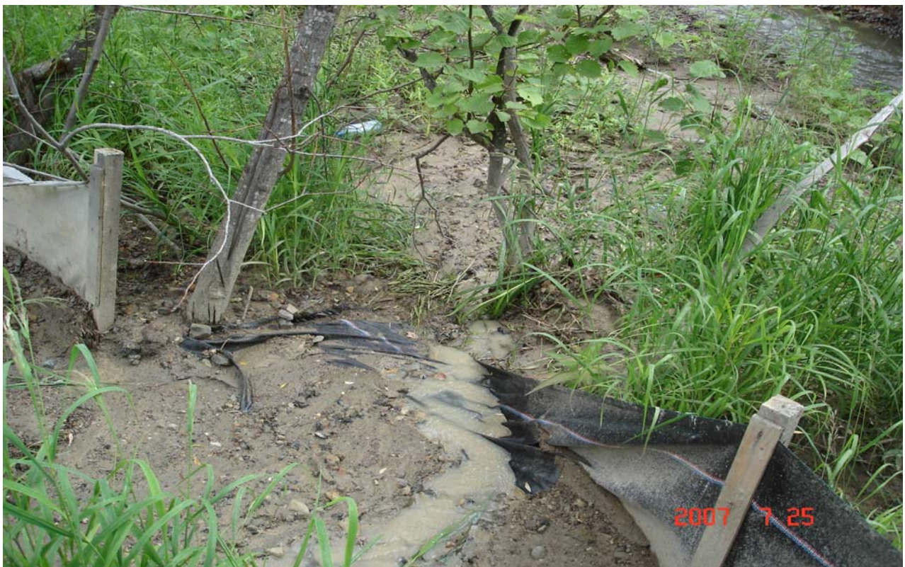
Right shore of the Krinka River, below the pipeline river-crossing. Running soil flows through the destroyed anti-sludge screens into the river.
