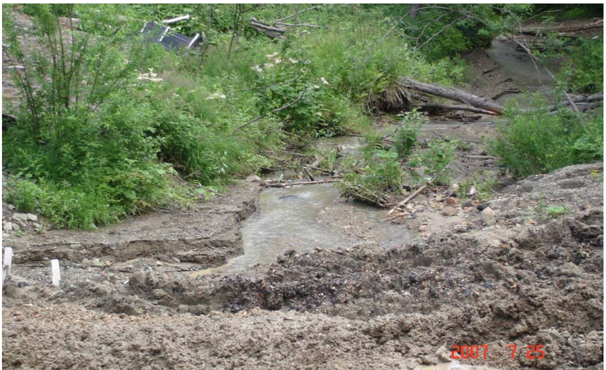
Un-numbered stream, KP 349.18. Downstream from the temporary bridge. Bank stabilization and anti-sludge screens are absent. As a result of the wash-out displaced into the stream and the slipping waste construction soil, the downstream water is very contaminated.
