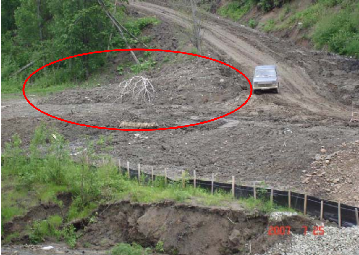
Right shore of the Krinka River. Disposal of easily-eroded waste construction soil on the protected shoreline zone of the river.
