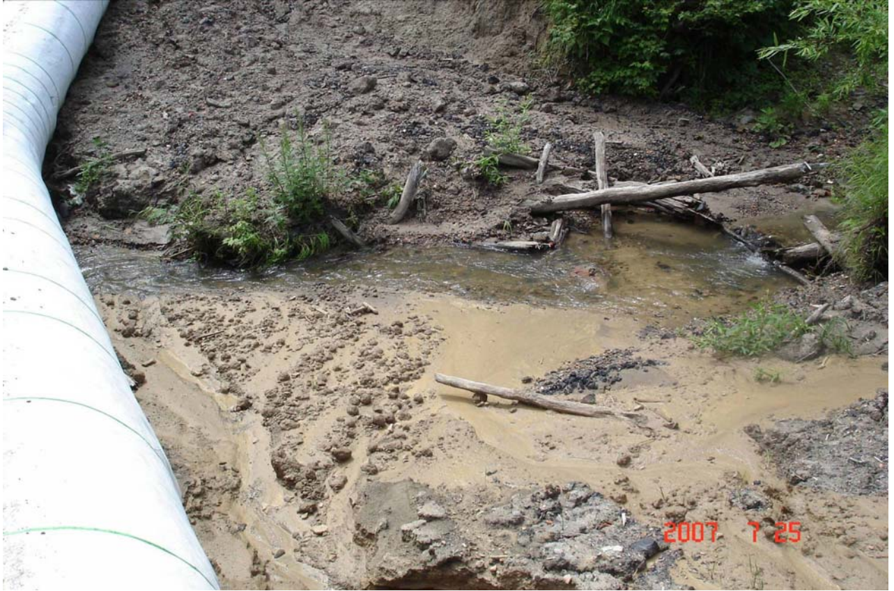
Un-numbered stream, KP 349.18. Upstream from the temporary bridge. Running soil from the pipeline route is slipping into the riverbed. Bank stabilization and anti-sludge screens are absent.
