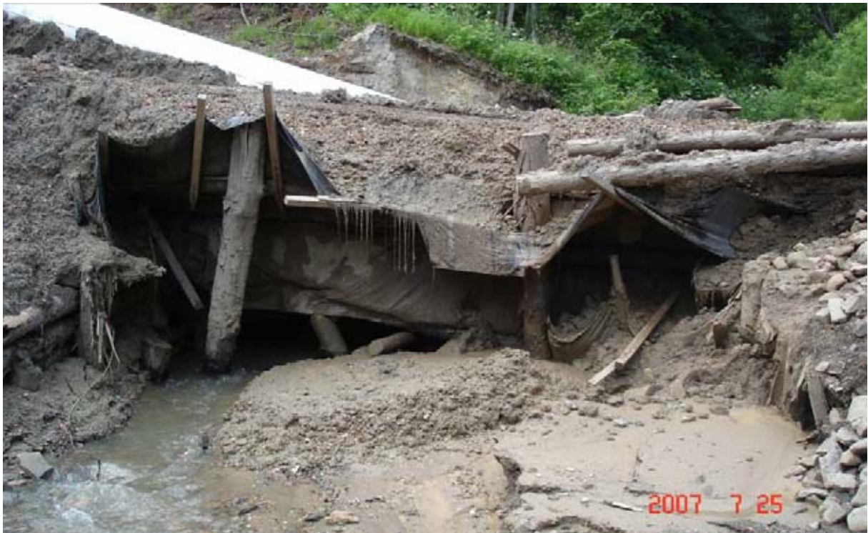
Un-numbered stream, right tributary of the Krinka River. KP 349.18. The bridge does not correspond to design requirements or matching conditions. The bridge supports have been built in the streambed. Waste construction soil is slipping into the streambed and being eroded by the water.
