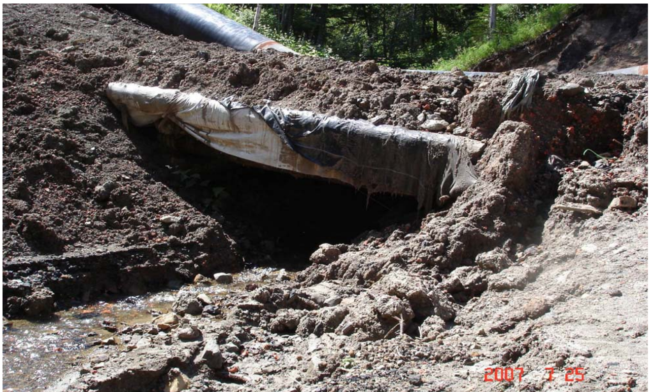
Petrovskii Stream, KP 351.1. The bridge does not correspond to design requirements and matching conditions. Waste construction soil is entering the streambed and contaminating the water.
