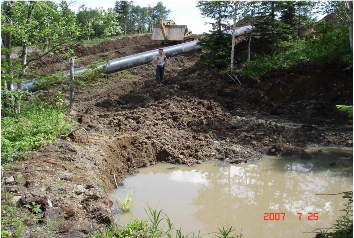
A section adjacent to the right-of-way, KP 350.6. Excavation of earth beyond the right-of-way, the destination of which the representatives of natural resource users could not explain.
