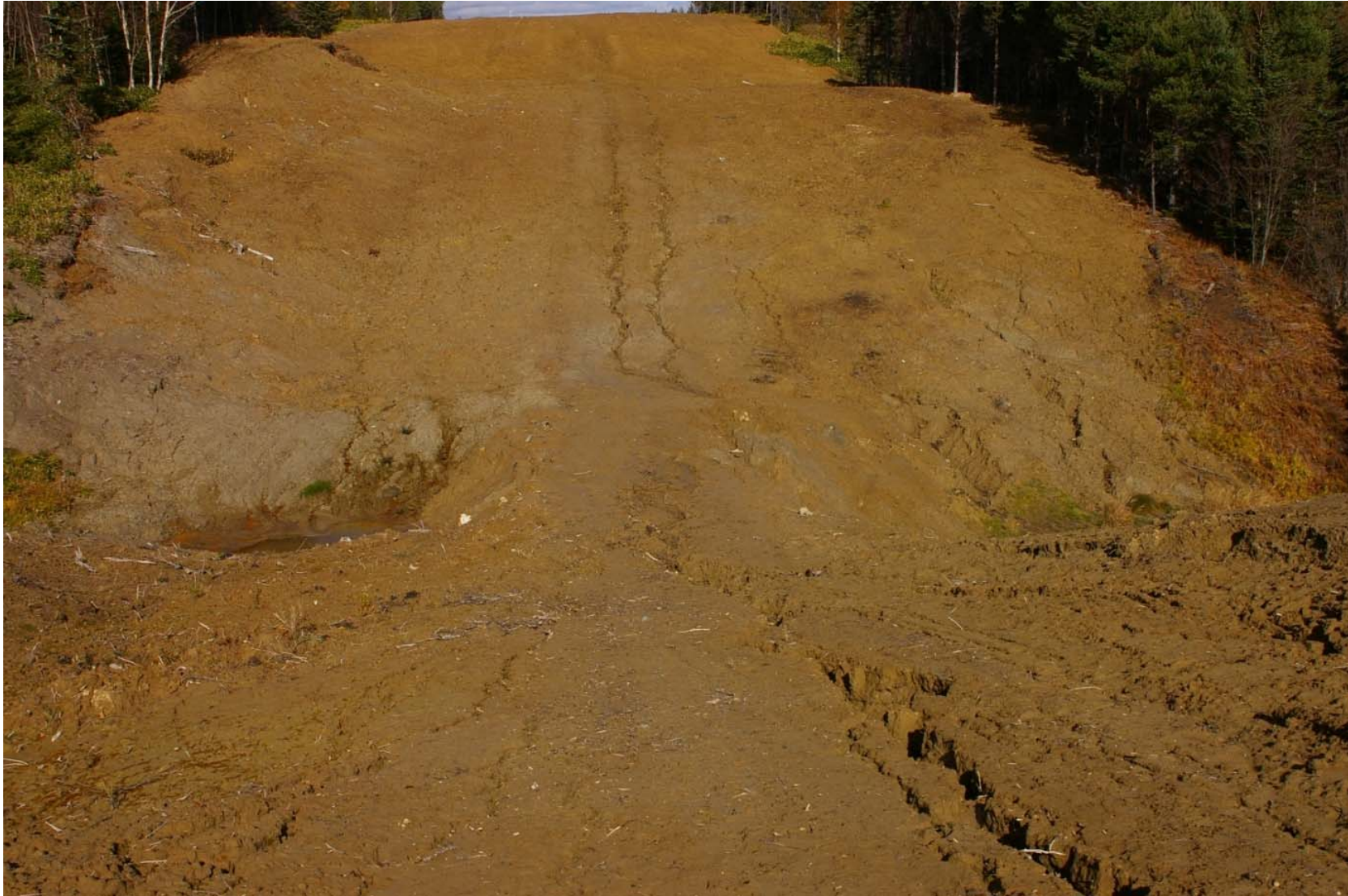
October 23, 2007: KP 490.2 Another stream to the north of the Krutoyarka River. This stream is also blocked by an earth mound which has been in place since last winter.
