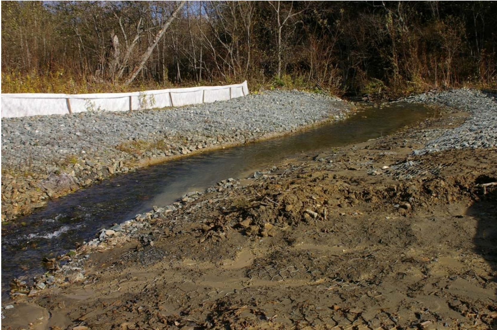
October 23, 2007: KP 482.5. The right bank of the Primorskaya River. SEIC doesn't maintain the Reno mats properly and doesn't have any land slide or erosion control measures in place on the adjacent slopes. As a result, sediments enter the river even during dry weather without the added effect of rainfall.
