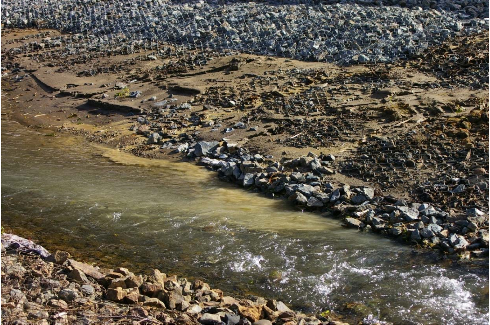
October 23, 2007: KP 482.5. The right bank of the Primorskaya River. Contamination of the river with soil runoff.
