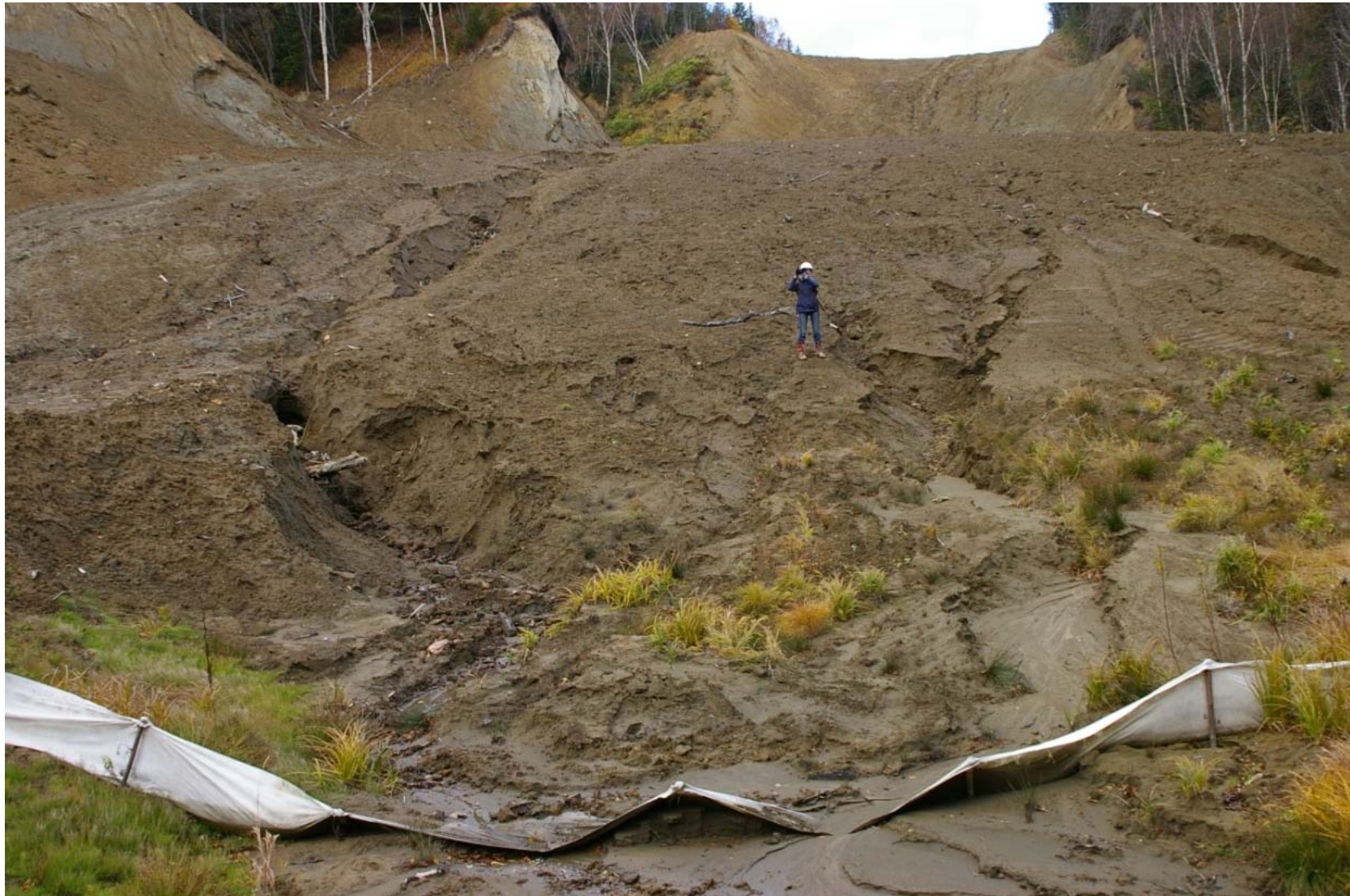
October 23, 2007: KP 492.5. Stream to the north of the Listvennitsa River (right bank). Massive, long term washout of earth into the stream is obvious.
