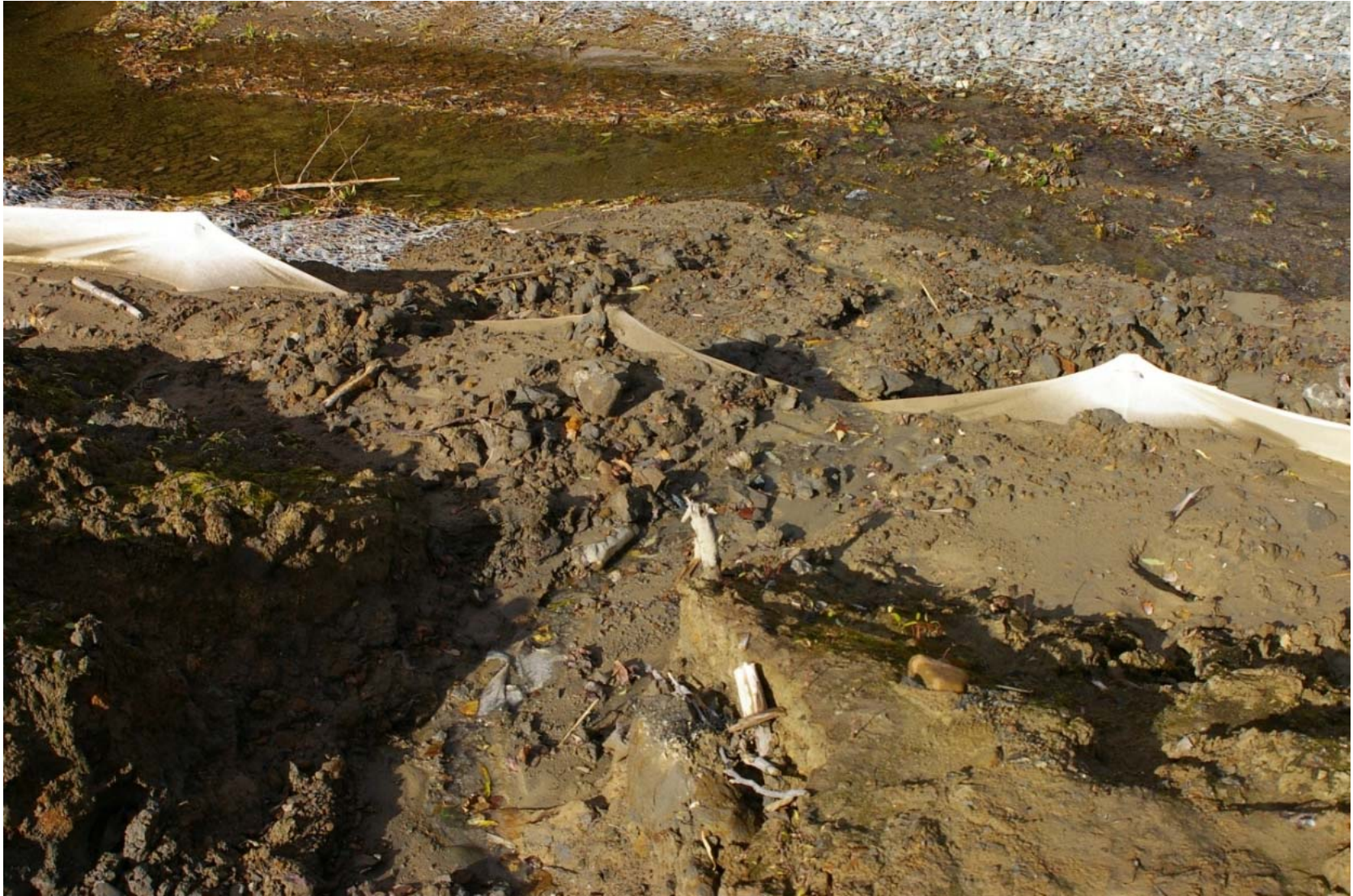
October 23, 2007: KP 491.4. Right bank of the Krutoyarka River. More failed silt fences.
