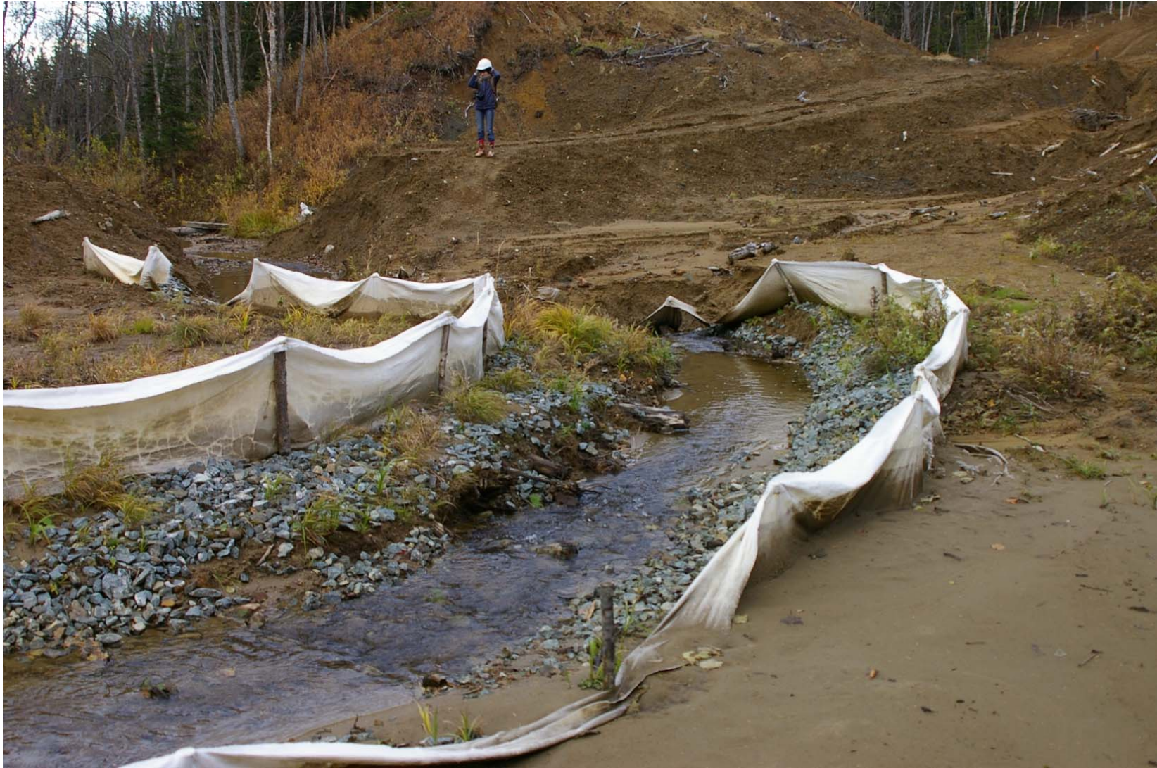
October 23, 2007: KP 493.7. The stream to the south of the Listvennitsa River. The stream has passed through an earth mound which was placed across the stream during "technical recultivation" last winter. The mound helped construction crews cross the stream during winter construction work. It's obvious that the mound in the background was placed after the silt fences were installed because the mound covers the silt fences. Since last winter nothing was done here to prevent or stop erosion or to maintain the stream and its tributaries.
