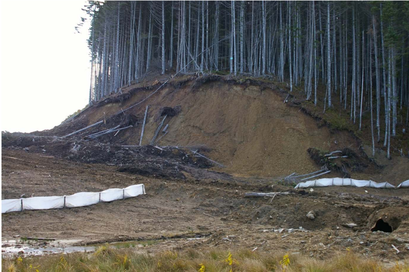
October 23, 2007: KP 483.7. Trees and soil have covered the RoW next to a stream to the north of Firsovo Village. There are no reinstatement measures.
