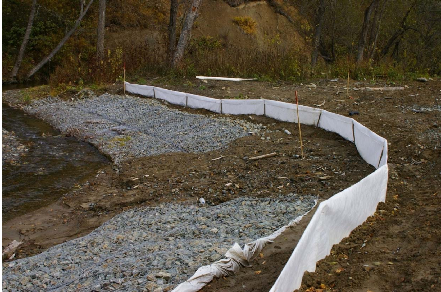
October 23, 2007: KP 489.5. The right bank of the Rybnaya River. Erosion trails over the Reno mat and into the river. A new silt fence was installed just recently over the erosion trail.
