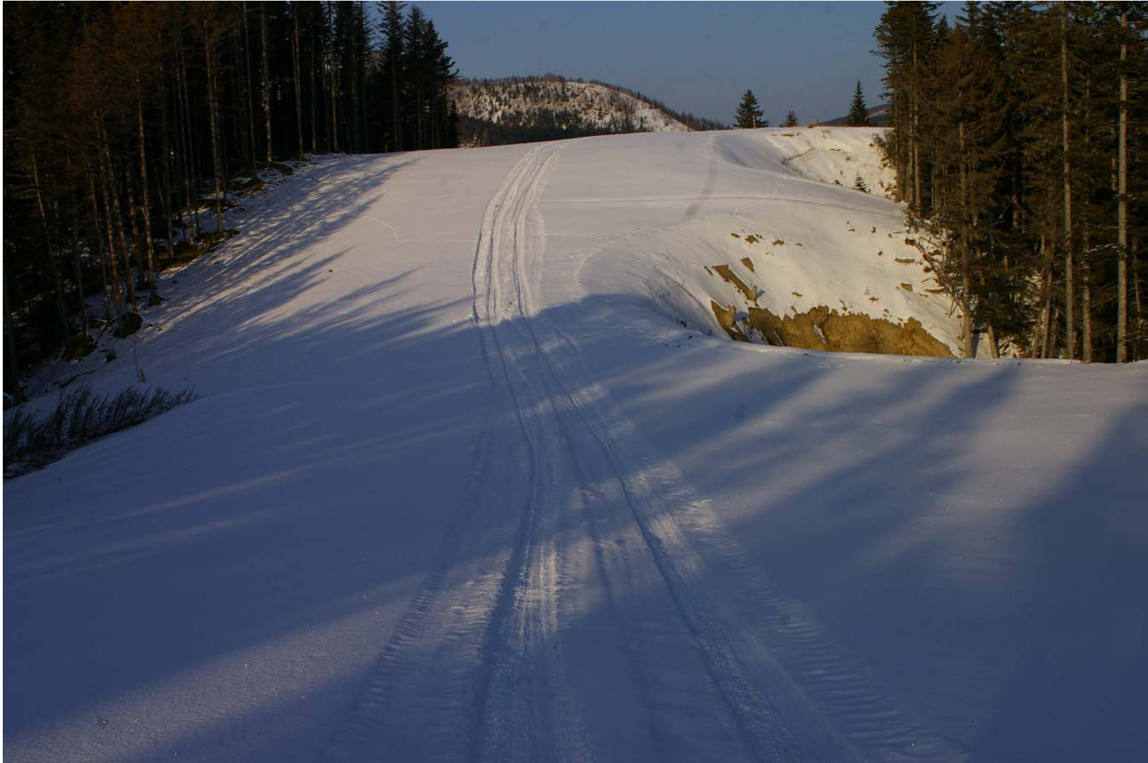
December 22, 2007: KP 365.1. A section of the pipeline to the north of the Pegas River crossing in Makarov District. The two washouts on the right appeared as a result of landslides. As spring approaches the threat of landslides will increase and erosion processes will undermine the oil pipeline here.
