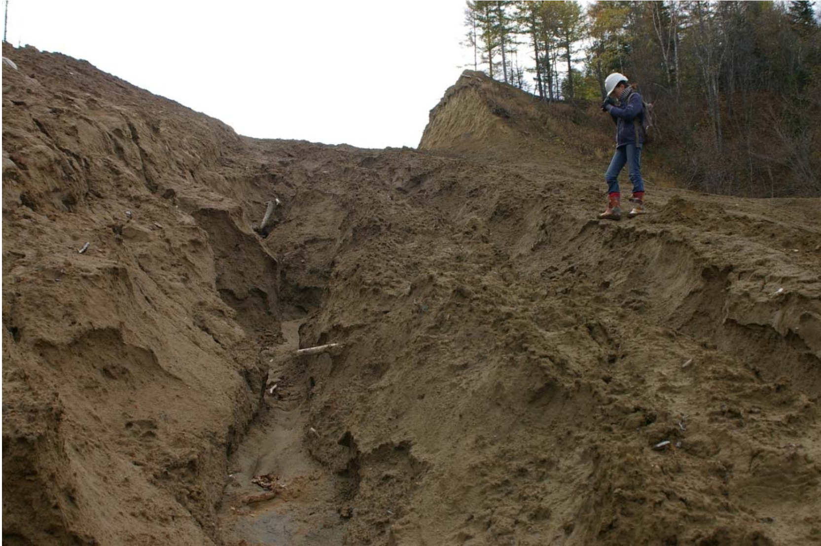
October 23, 2007: KP 492.5. Stream to the north of the Listvennitsa River (right bank). Very deep erosion ditch on the pipeline RoW.
