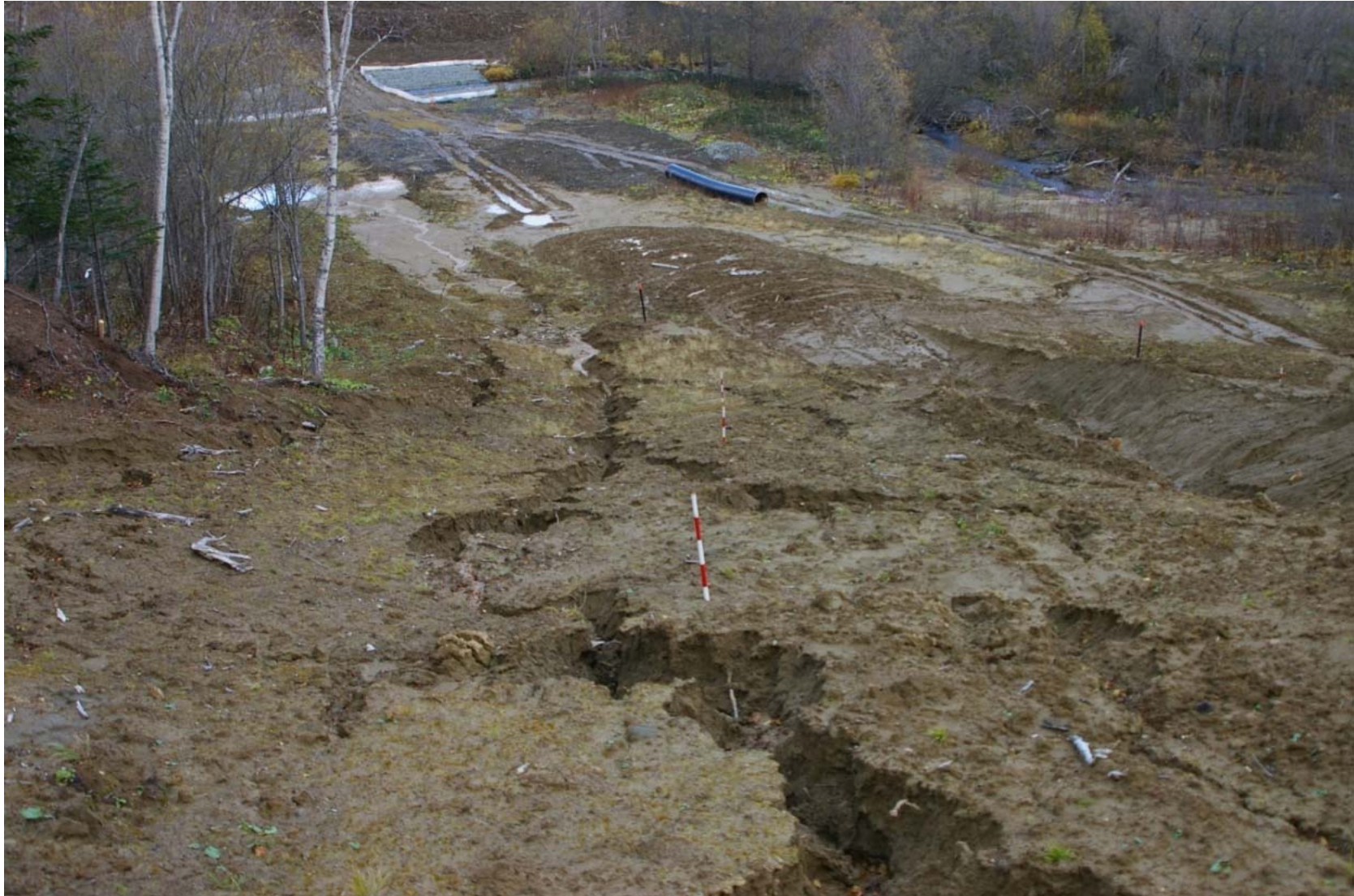
October 23, 2007: KP 492.9. Right bank of the Listvennitsa River. Erosion ditches on the pipeline RoW.
