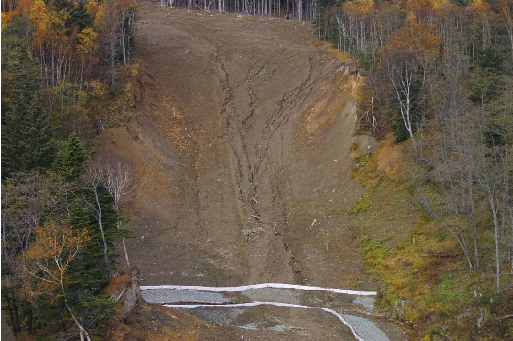
October 23, 2007: KP 489.5. The Rybnaya River and its left bank. Erosion trails over the Reno mat. The silt fences were installed just recently, over the erosion trails.
