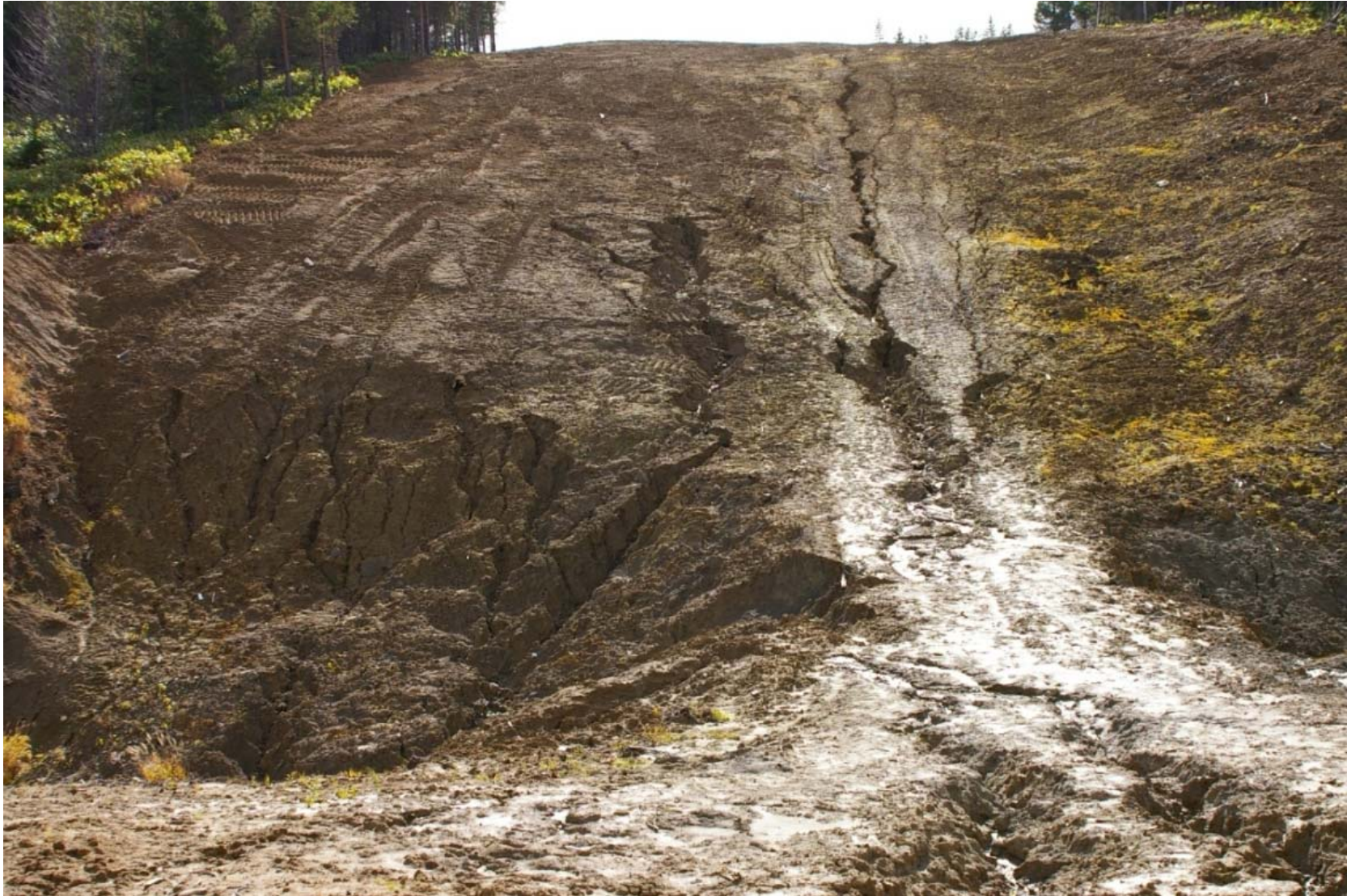
October 23, 2007: KP 490.2. Another view of the second stream to the north of the Krutoyarka River which has been blocked by an earth mound since last winter.
