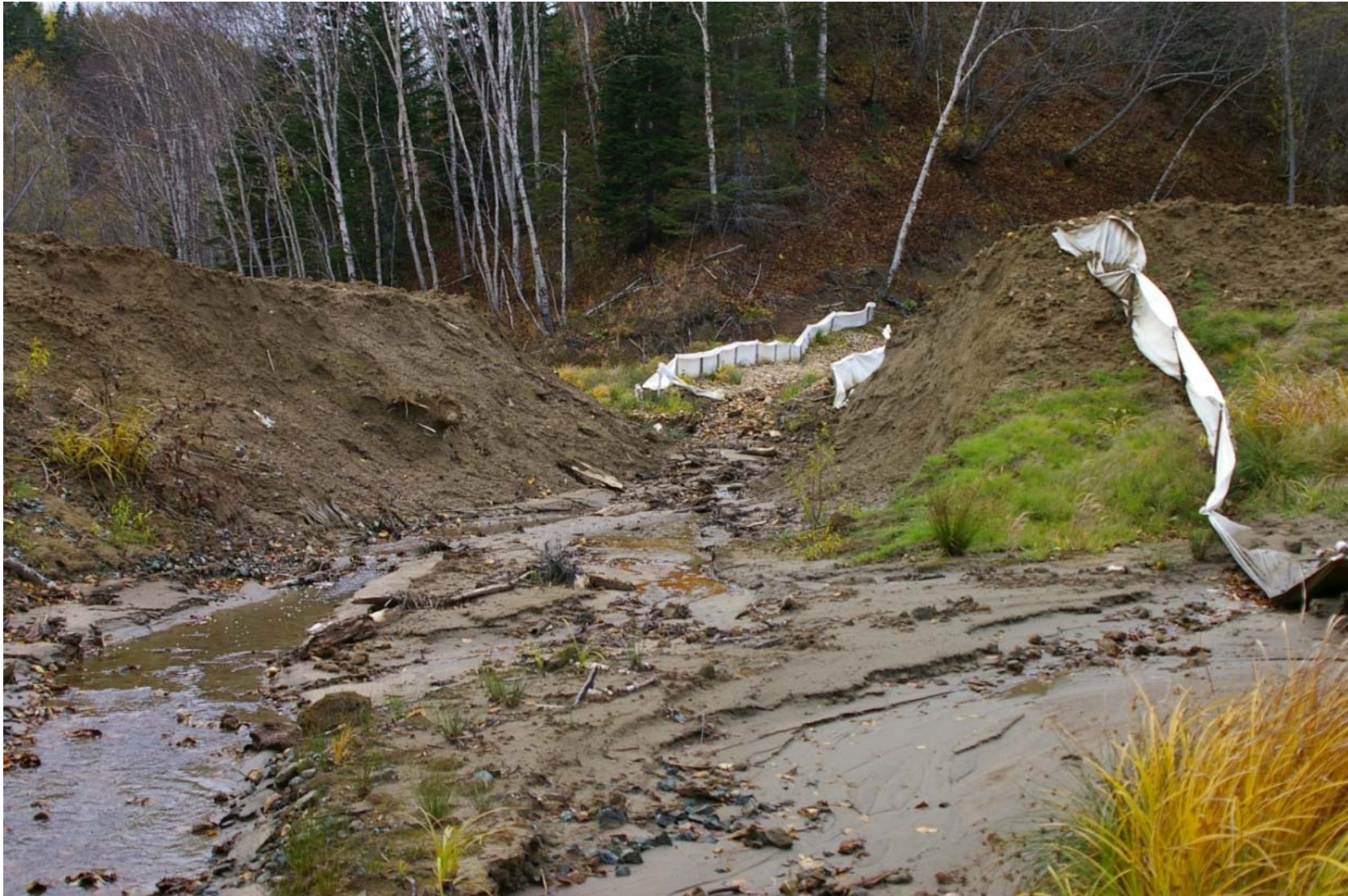
October 23, 2007: KP 492.5. Stream to the north of the Listvennitsa River. Again, the stream has passed through an earth mound which was placed across the stream during winter "technical recultivation," creating a source of erosion into the stream. Tens of tons of earth were washed into the stream.
