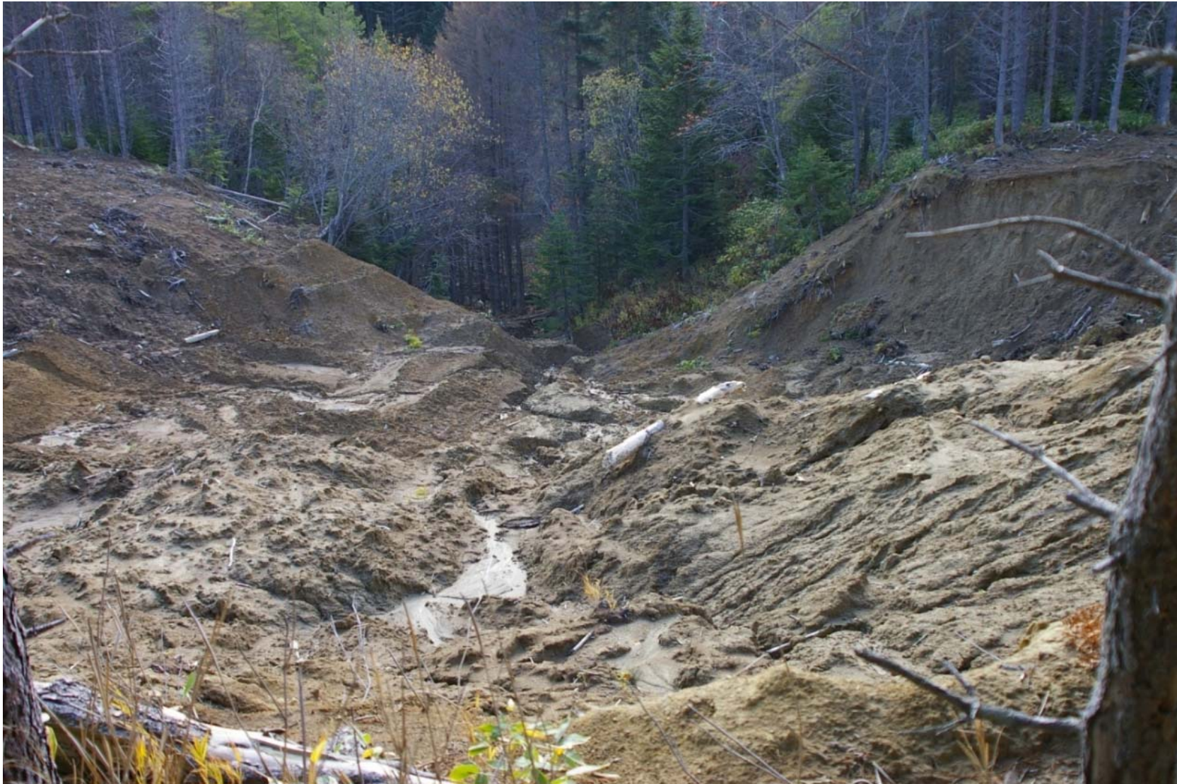
October 23, 2007: KP 483.3. To the north of Firsovo Village. A deep erosion canyon across the pipeline RoW.
