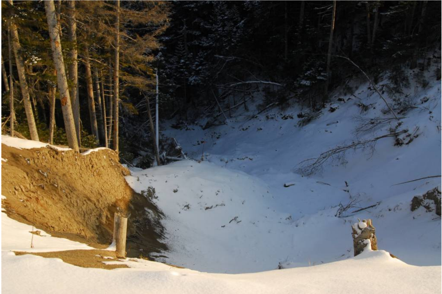
December 22, 2007: KP 365.1. A section of the pipeline to the north of the Pegas River crossing in Makarov District. A landslide down the hill from the pipeline RoW.
