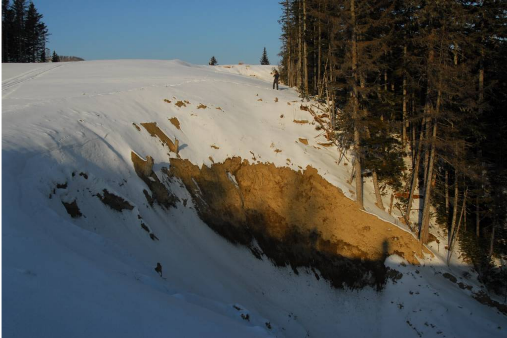
December 22, 2007: KP 365.1. A section of the pipeline to the north of the Pegas River crossing in Makarov District. A landslide zone which undermines the pipeline is pictured.
