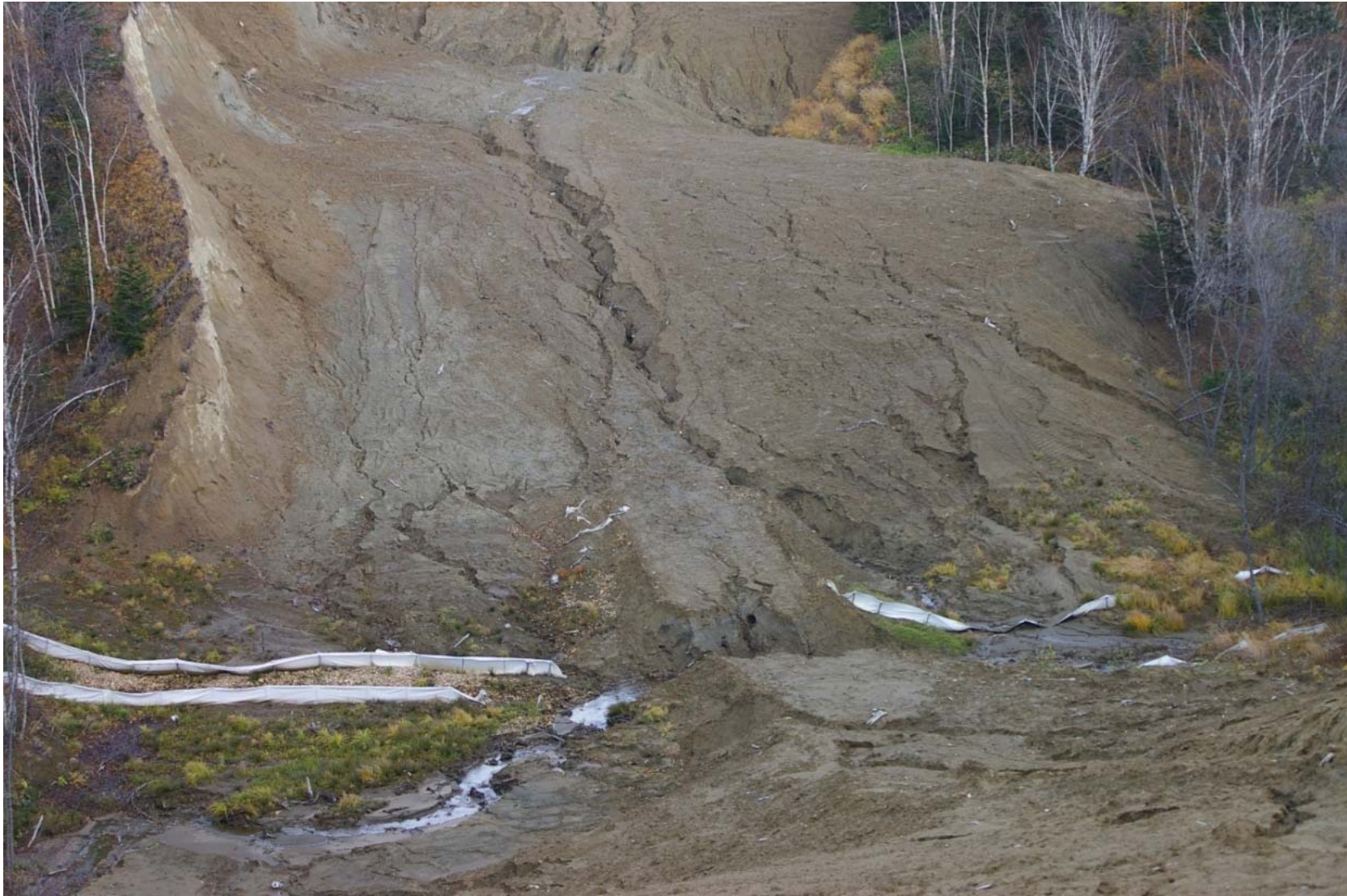
October 23, 2007: KP 492.5. Stream to the north of the Listvennitsa River (left bank). Erosion ditches on the pipeline RoW. The stream has made a channel through the earth mound placed across the stream last winter. The earth mound (here and in other locations) was made for vehicles which were doing "technical recultivation" last winter. The main purpose of the mound was to simplify stream crossings for vehicles during winter operations, yet this "technical recultivation" is now a source of erosion into the stream.
