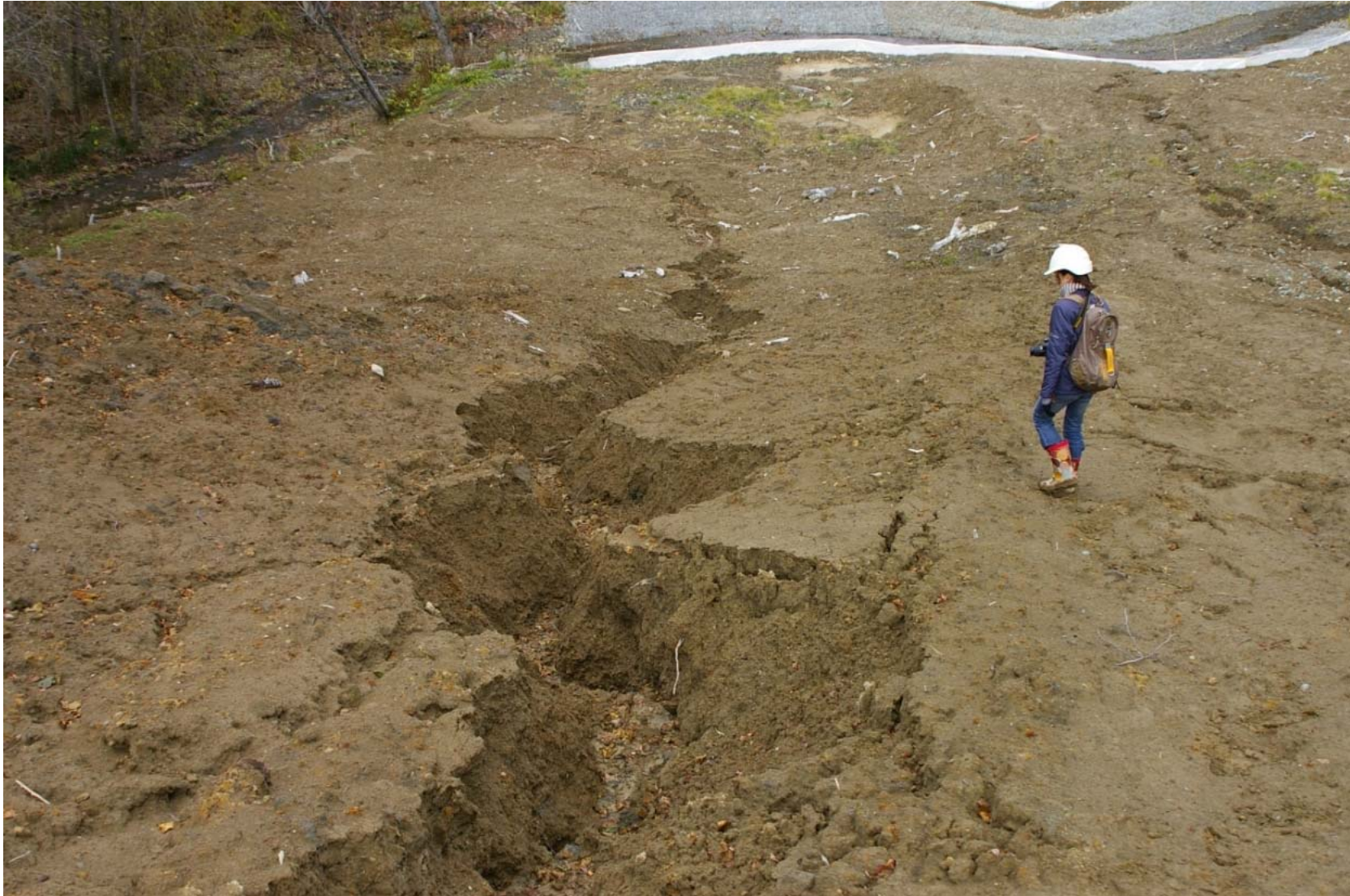
October 23, 2007: KP 489.5. Erosion trench flows down the right bank of the Rybnaya River unabated by erosion control measures.
