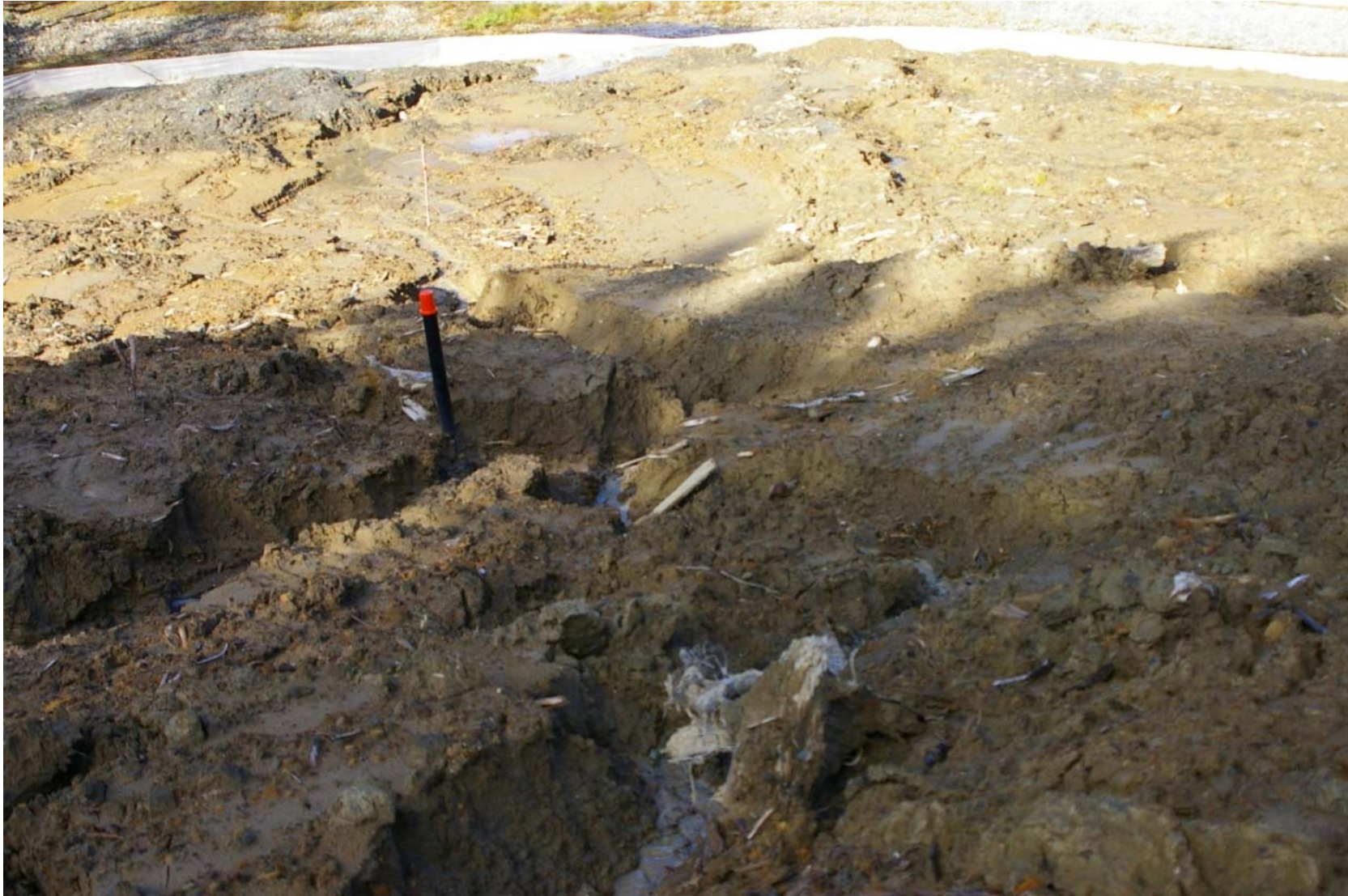
October 23, 2007: KP 482.5. The right bank of the Primorskaya River. Erosion is taking place directly above the gas line. The black stick with the orange cap is a cathode protection check point.
