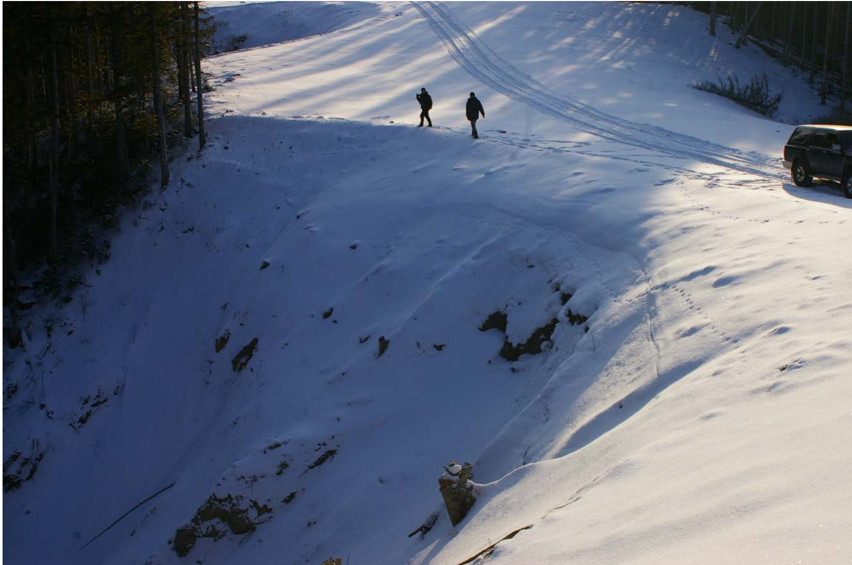
December 22, 2007: KP 365.1. A section of the pipeline to the north of the Pegas River crossing in Makarov District. A landslide zone which undermines the pipeline is pictured.
