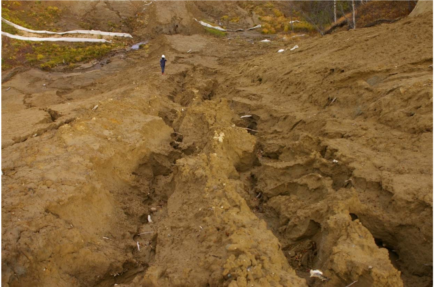
October 23, 2007: KP 492.5. Stream to the north of the Listvennitsa River (right bank). Severe erosion ditches on the pipeline RoW.
