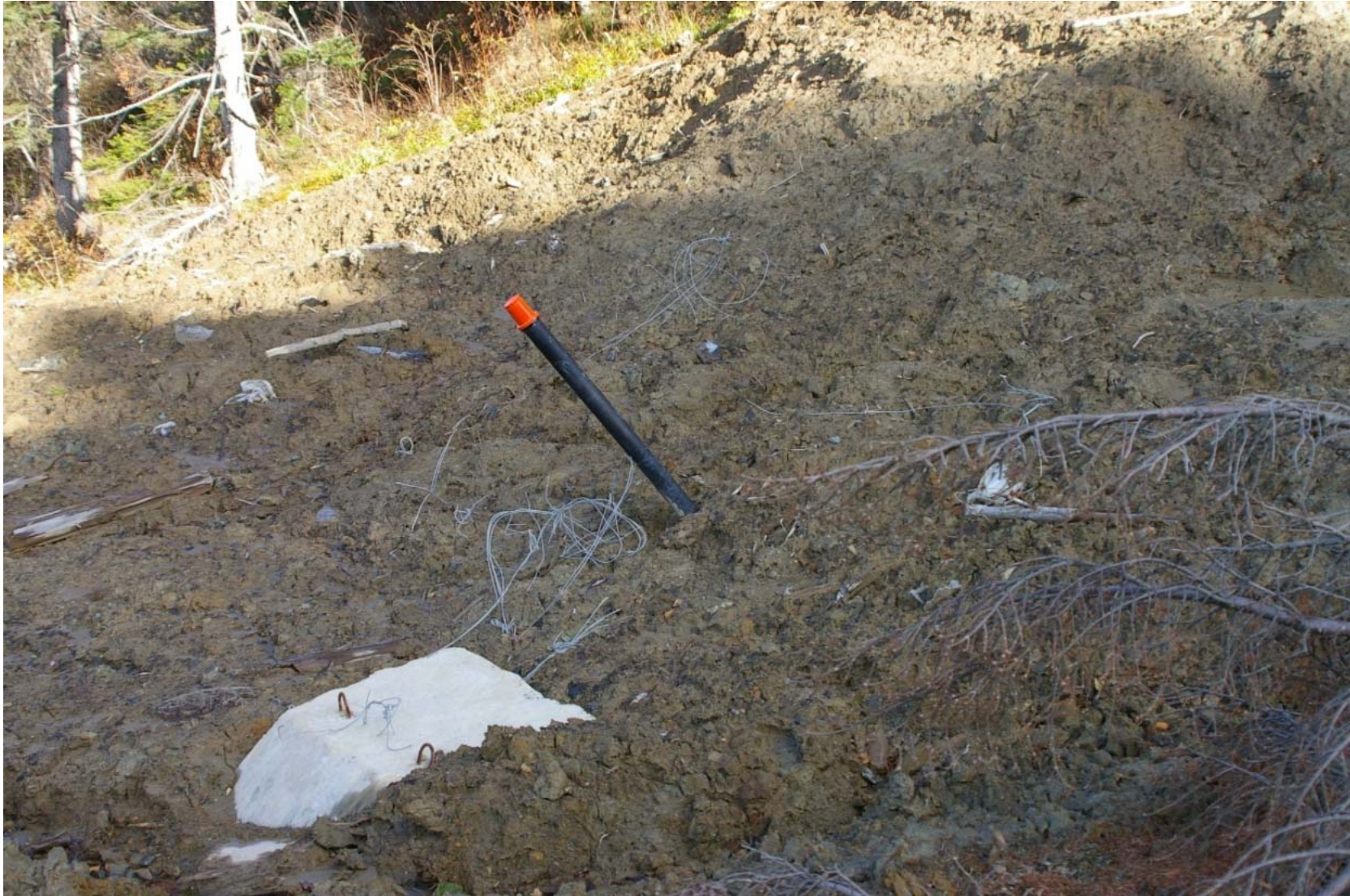
October 23, 2007: KP 482.5. The right bank of the Primorskaya River. The cathode protection check point for the oil line has been broken by the creeping land slide.
