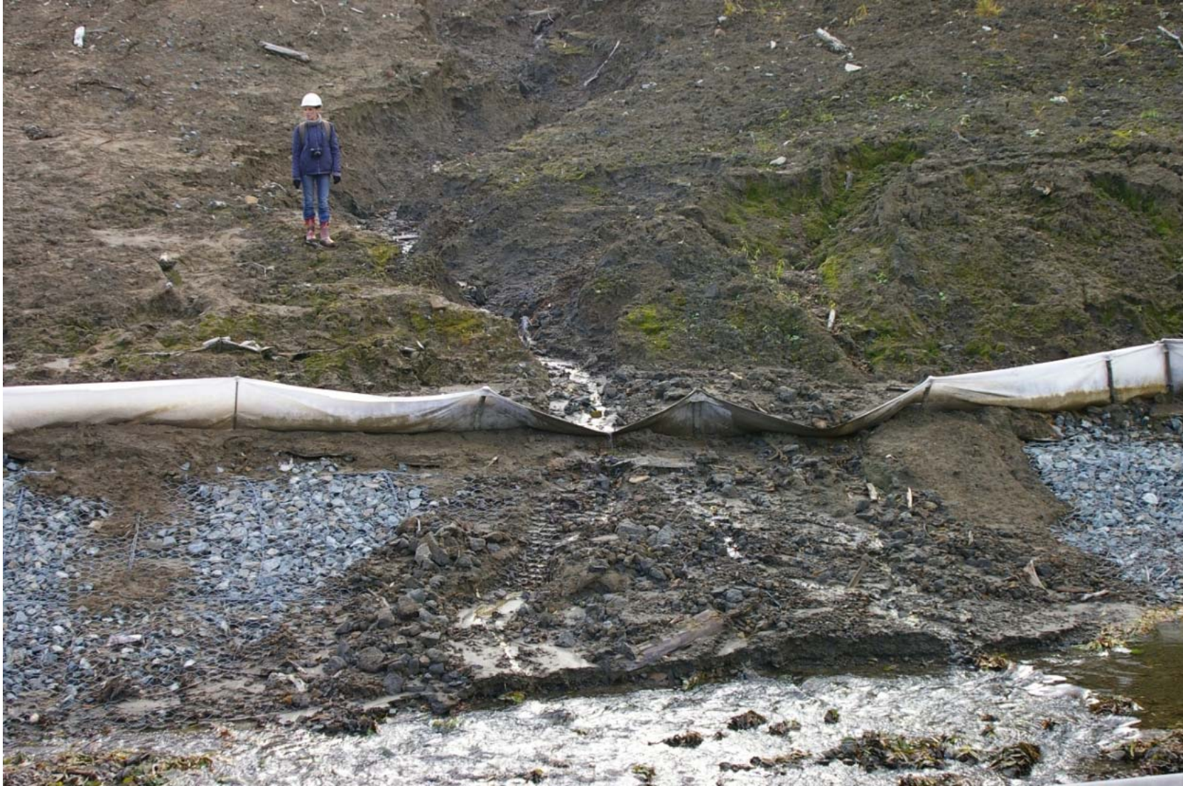
October 23, 2007: KP 491.4. Right bank of the Krutoyarka River. The silt fences don't work and erosion runoff enters the stream.
