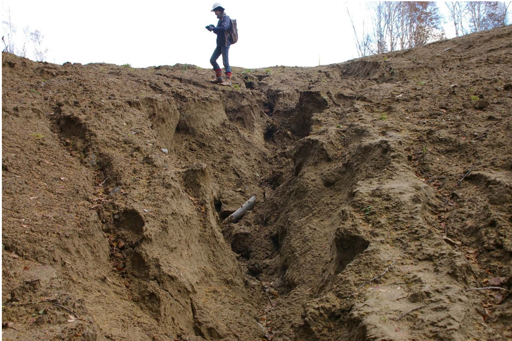
October 23, 2007: KP 493.2. 300 meters to the south of the Listvennitsa River. Very deep erosion ditch on the pipeline RoW.
