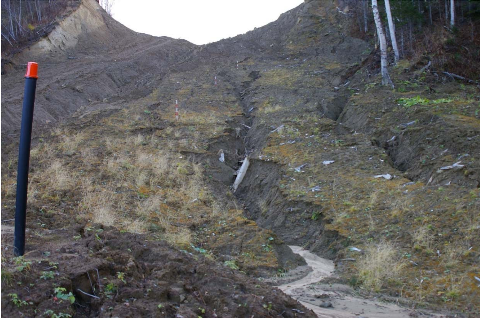
October 23, 2007: KP 492.9. Right bank of the Listvennitsa River. Erosion ditches on the pipeline RoW. This stream is muddy brown from erosion runoff.
