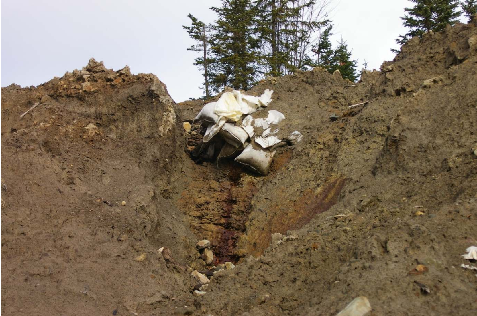
October 23, 2007: KP 490.5. Left bank of the stream to the north of the Krutoyarka River. Failed anti-erosion and anti-land slide measures. Though a very few anti-erosion measures such as this were observed, they absolutely failed to achieve their intended purpose.
