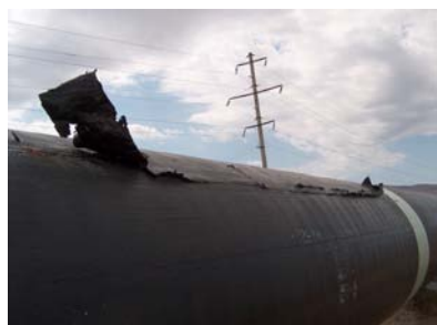
Damaged Pipe in Rustavi
