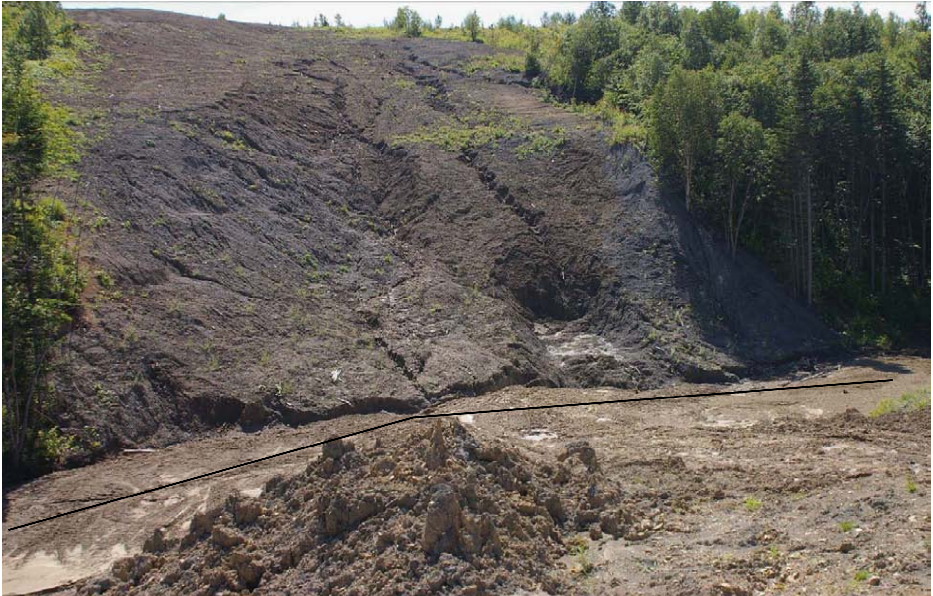
PK 462.6. A section of the route in the crossover point over the left tributary of the Baklanovka River (flows into the Sea of Okhotsk). Dolinsk District. Again, the typical situation where landslides of various scales are being formed. The line marks the former streambed which is now completely overwhelmed with the sediment drifted down. The need for urgent remediation work is obvious. August 31, 2007.
