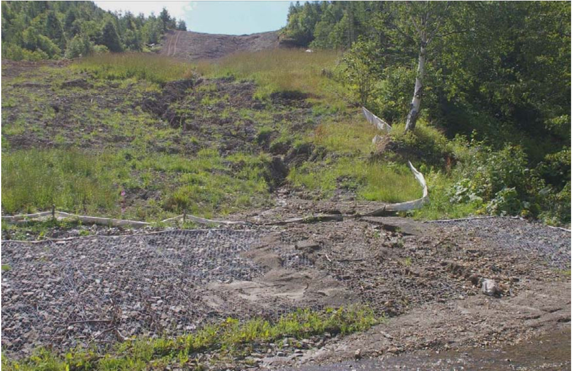
PK 460.2. A section of the route crossing over the Krasnaya River (the right bank). Dolinsk District. The active gully and the outwash tail of the soil to the riverbed – right over the bank protection structures – may well be seen in the foreground. August 31, 2007.
