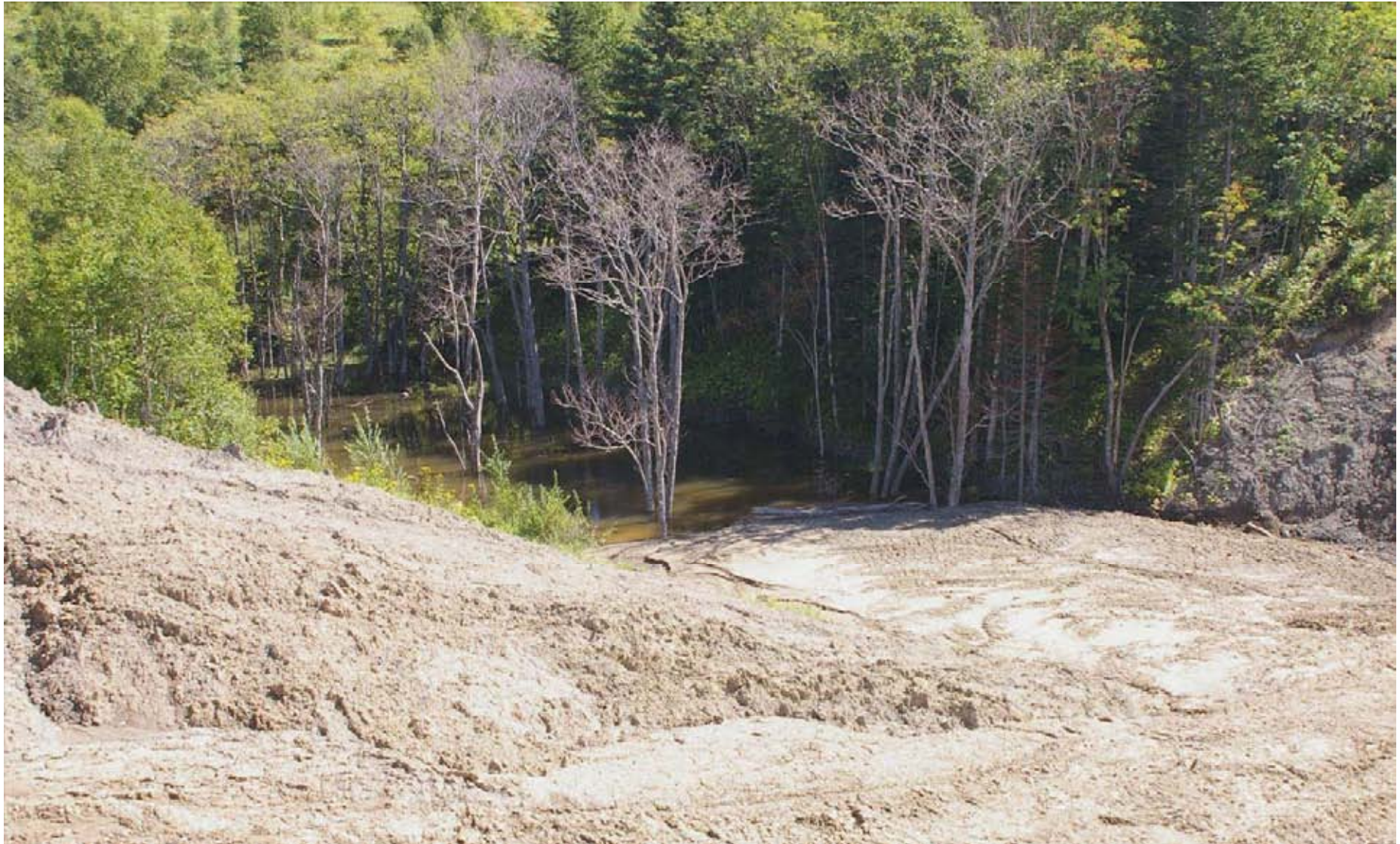
PK 462.6. A section of the crossing over the left tributary of the Baklanovka River. Dolinsk District (the same site as the one on the preceding slide). A massive landslide blocked the riverbed having completely disturbed the hydrologic characteristics thereof. The trees in the stream floodplain are dying as a consequence. August 31, 2007.
