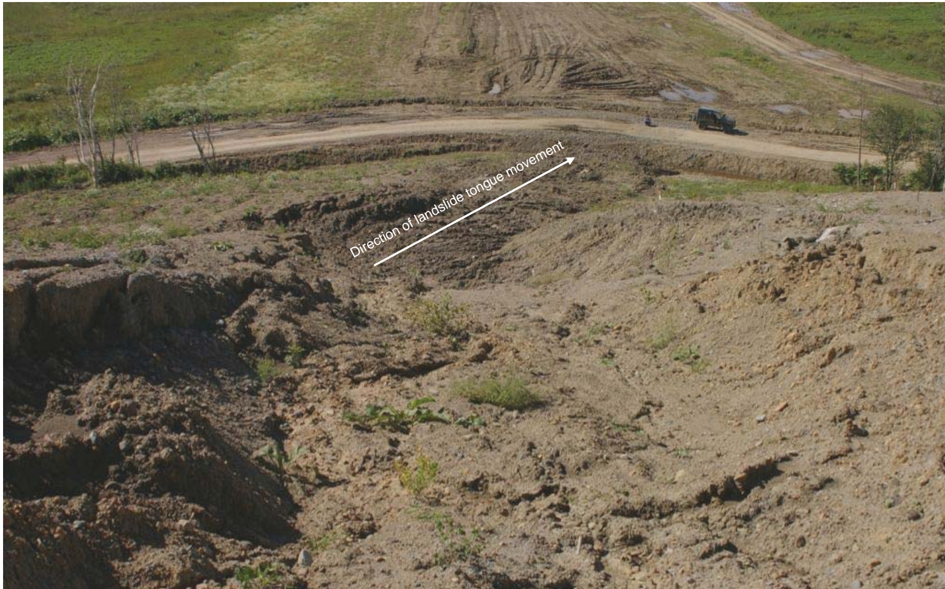
PK 504.7. A section of the route to the north from the Ay River. Dolinsk District. (the principal site of the inspection conducted in October 2006 by the Committee of the Ministry of Natural Resources of the Russian Federation). The situation here has but gone from bad to worse, in spite of the fact that on August 8, 2007 an inspection was conducted here by the Federal Service for Supervision of Natural Resource Usage in Sakhalin Region and directives were issued regarding the elimination of the violations. The mud flow continues in development making the trench over the installed pipes deeper and carrying the bulks of soil into the stream, a tributary of the Ay River, flowing beneath the hillside. August 31, 2007.
