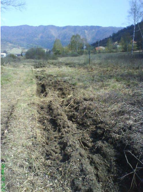
Pict. 2 Shrub debris, sod removal and the planned extension of the digging route of the trench along the northern border of Rojkovské Rašelinisko Mire Nature Reserve (view to the east, 24th April 2010)
