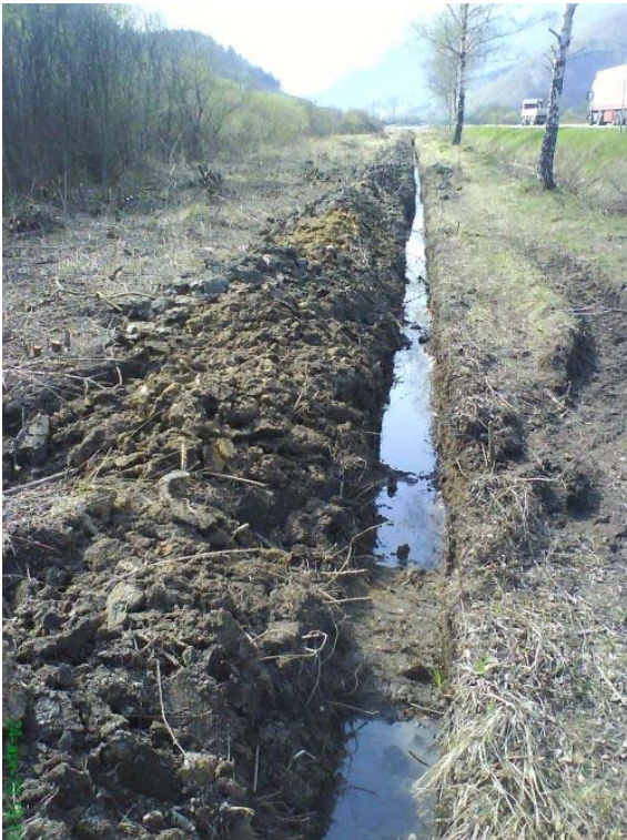
Pict. 1 Dig off of the trench for relocating a cable, draining the northwest part of the Rojkovské Rašelinisko Mire Nature Reserve (view to the west, 24 th April 2010)
