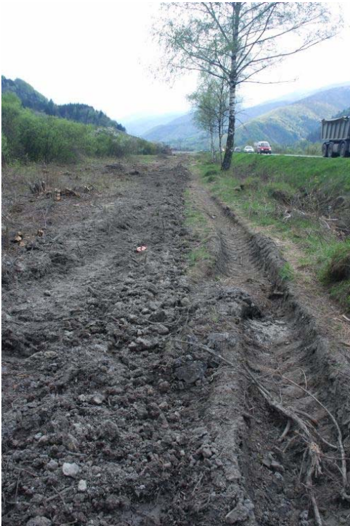
Pict. 4 Filled in trench along the northern border of Rojkovské mire (1 st May 2010)
