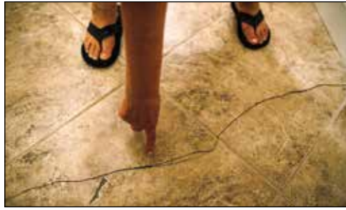
Mary Mahan, a resident of Greenbier, points to a crack in the floor tile of her home that was a result of an earthquake.
