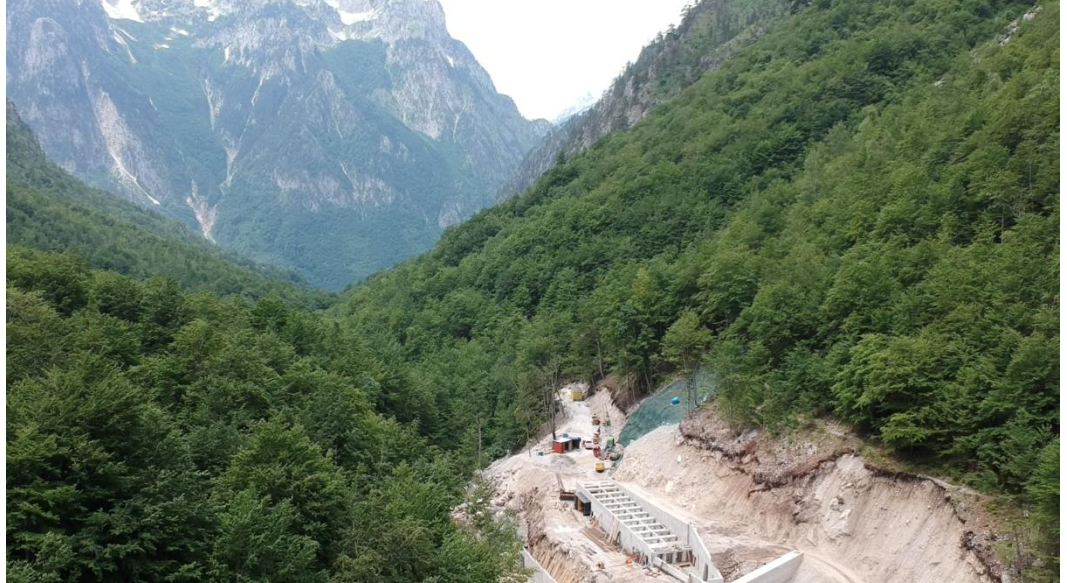
Hydropower construction in the Valbona Valley National Park, Albania, is one of many egregious examples of biodiversity destruction in the Energy Community countries. Photo: David Hoffman
