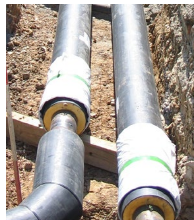
District-heating-pipeline made of preinsulated bonded pipe systems
