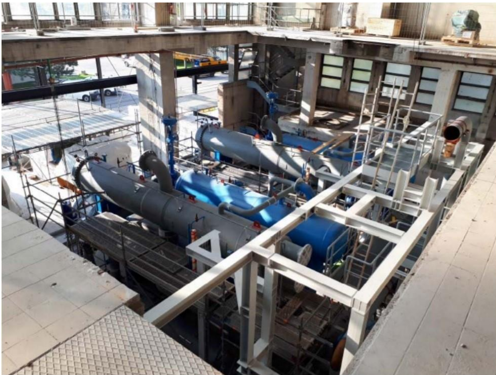
Figure 1: View of the large heat pump in Wien Simmering (source: Segalla, 2018). ©Wien Energie / Zinner
