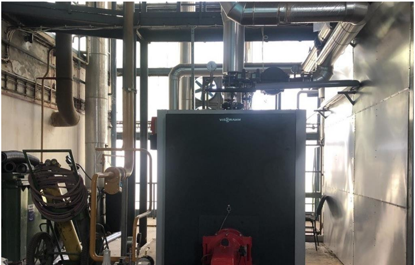
Geothermal water plant in Szeged, Hungary with new, more efficient radiators for local residences
