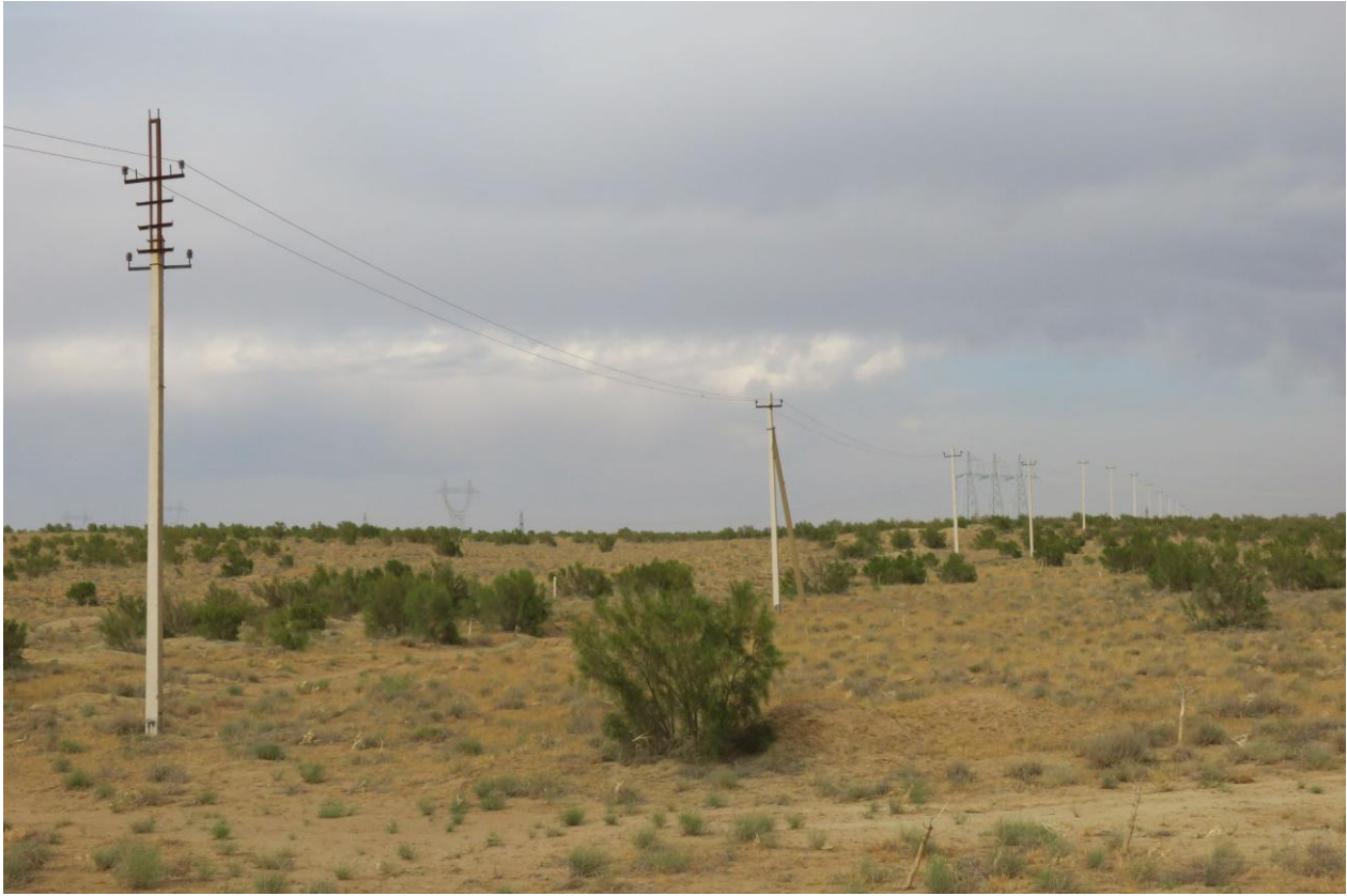
"Killer" type mid-voltage power line poles at Bash wind project area (©CEE Bankwatch Network)
