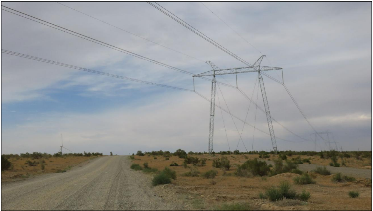
Transmission line at Bash wind project with no bird diverters (©CEE Bankwatch Network)
